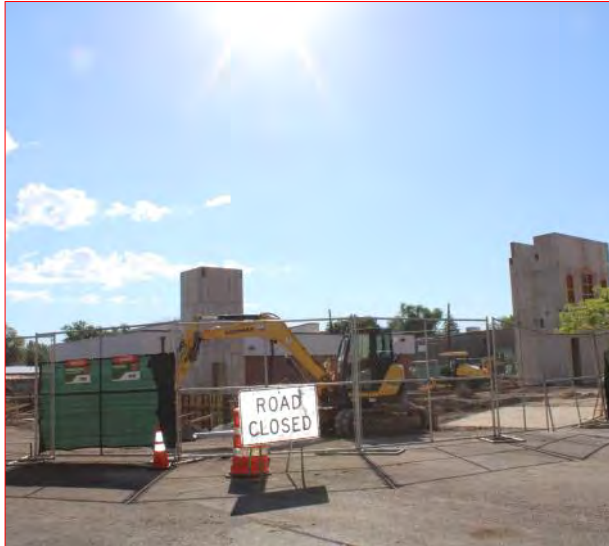
Measure 2A helped to fund a new police facility, now under construction, above. Mirror file photo.
